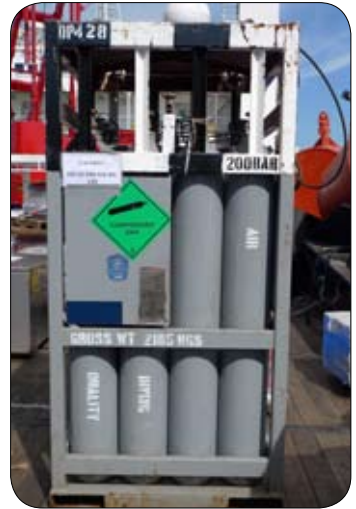
Photo 20: Typical HP air quad.
