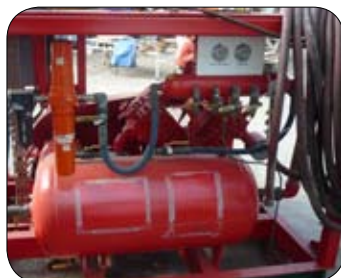
Photo 18: Typical LP air compressor.
