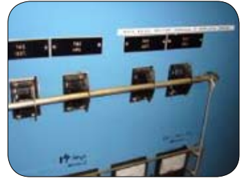
Photo 2 : Lock Out/Tag Out notice on ship equipment panel.
